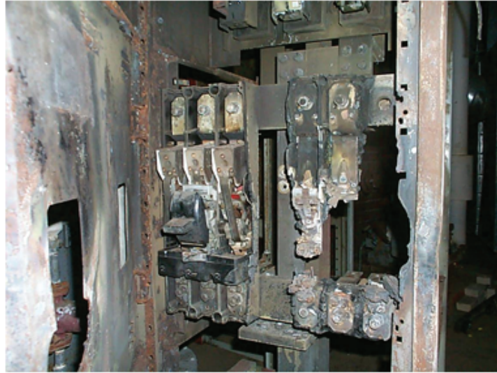
Figure 92 - Example of Arcing Damage to Equipment
