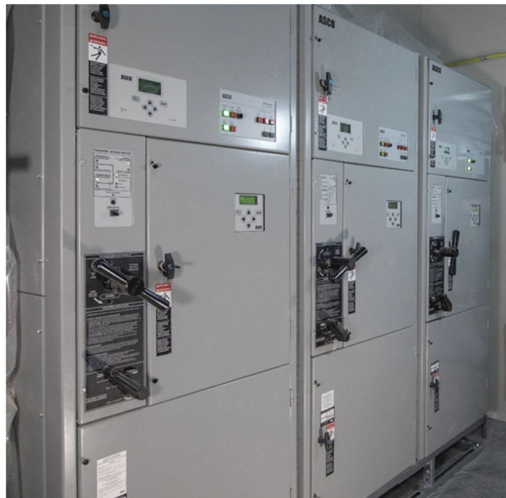
Figure 114 - Automatic-transfer- Bypass/isolation Switches
