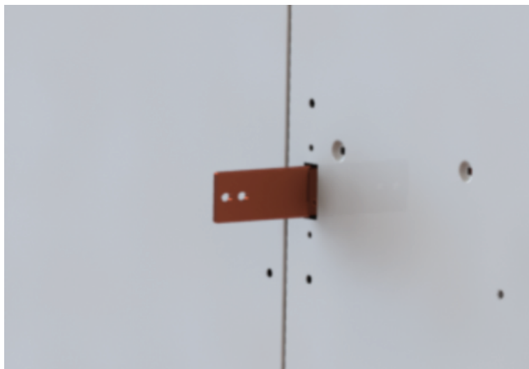
Figure 41 Connecting Point of Switchgear Earth Bus to Building Earth
