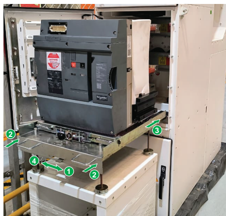
Figure 27 Move trolley with circuit breaker towards the panel until they are in contact, and lock.
