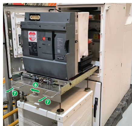
Figure 26 Extracting the Circuit Breaker onto Trolley
