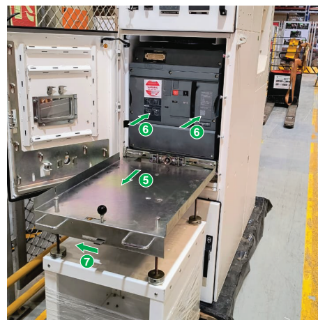
Figure 28 Pushing the circuit breaker into the panel.
